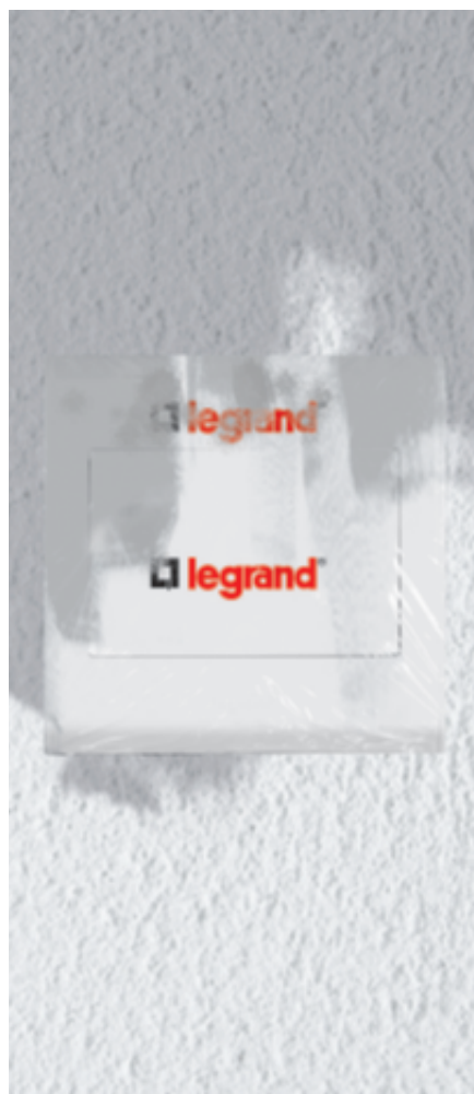
Only the soft protective film will get stained by the ongoing wall paintwork.
